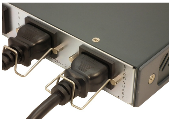
Figure 3-7 AC Power Input
